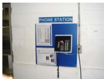
Example of a Phone Station
